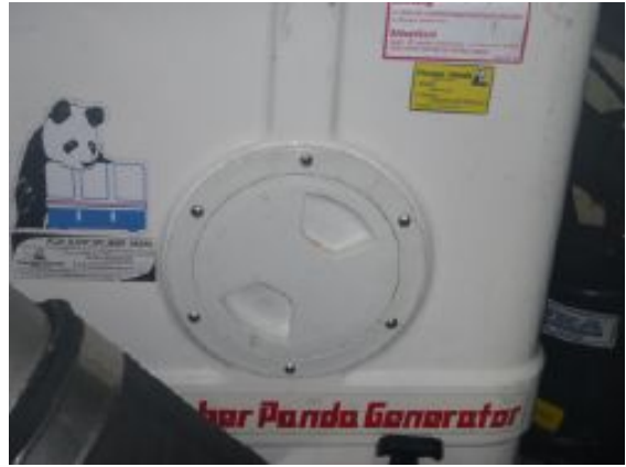
> 8KW Panda Generator 1158 Hours
