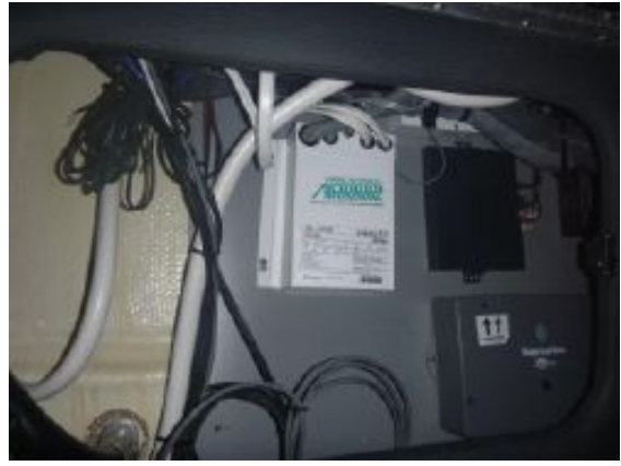
> Electrical Access in Mid Cabin
