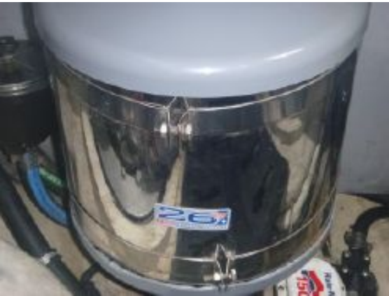
> Hot Water Heater
