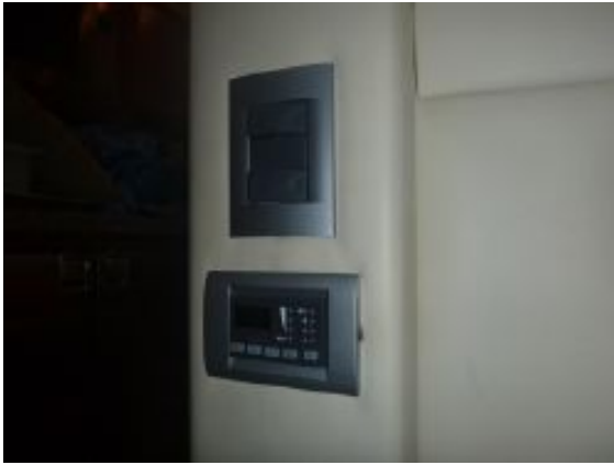
> Mid Cabin A/C Panel
